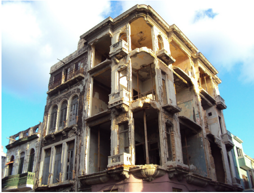
A collapsed building near Old Havana 6
