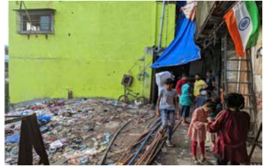
Figure 4: Cables forming improvised connections to utilities running through a street in Behrampada.
